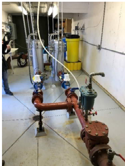
FIGURE 5 – WATER TREATMENT FACILITY INTERIOR
