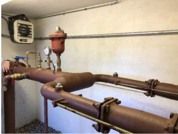
FIGURE 3 – WELL CONTROL HOUSE INTERIOR road.
