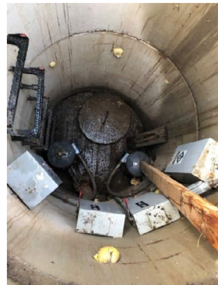
FIGURE 2 – INFILTRATION GALLERY DRY PIT INTERIOR
