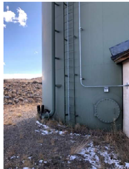
FIGURE 7 – UNSECURED LADDER ON WATER STORAGE TANK
